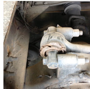
Bushing Material Is Torn Or Cracked
